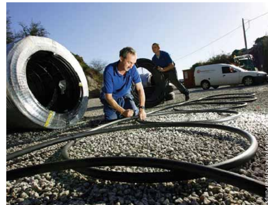
Groundsource heat pump installation
